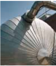
Energy storage Cristopia
